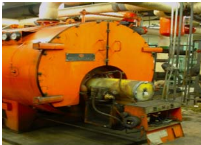
Evaluation of 250 HP, Oil Fired, Hot Water Boiler Following Fire Damage from Failure of Fuel Oil Metering Valve
